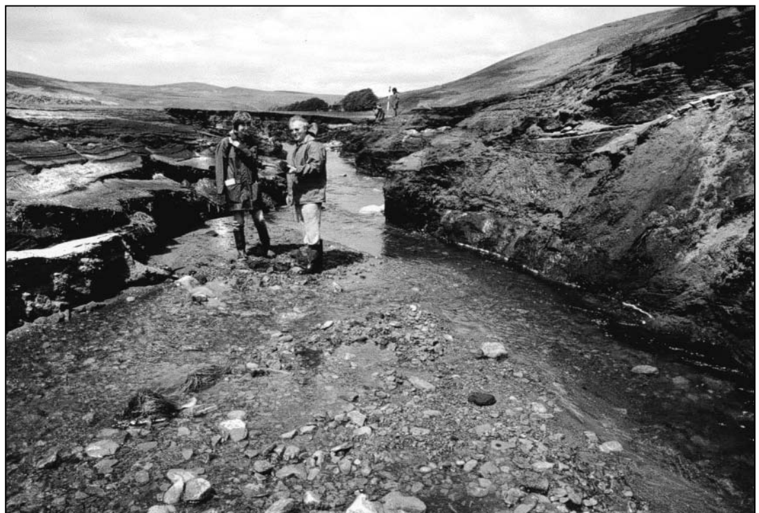
Figure 7. Channel cut through sediments in Wessenden Old Reservoir, Yorkshire, when it was drained for repair works.
